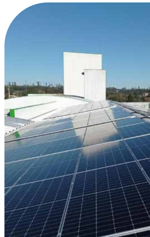
A production unit with 362 photovoltaic panels, each with a capacity of 550 Wp, has been installed at the Santa Comba Dão site in Portugal.
